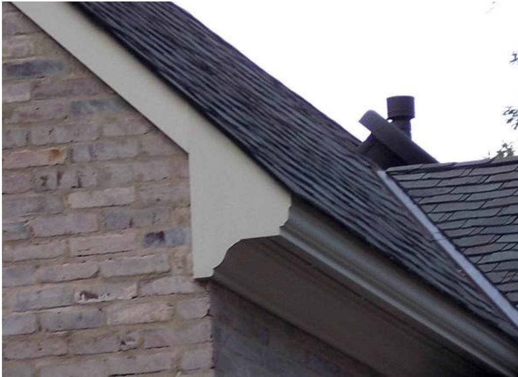
PROFILE - Flush Rake with decorative cornice end board as a molding stop
